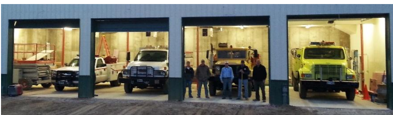
Station 1 interior work showing four of the five bays, January 2015. As with all construction projects, RCVFD volunteers contributed considerable time and effort into making the project a reality.
